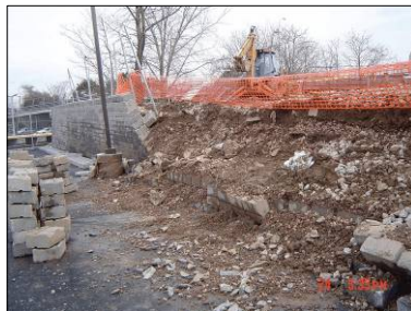
Forensic Evaluation - Retaining Wall Failure
